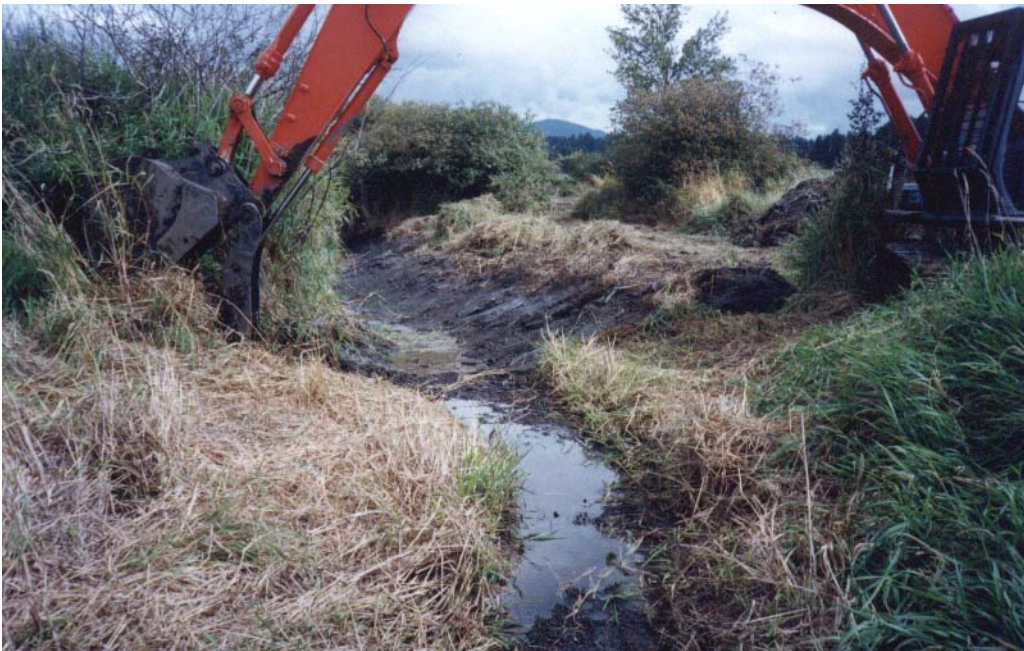
Photo 4: The channel sections were excavated with a 245 class excavator with a cleanup bucket
