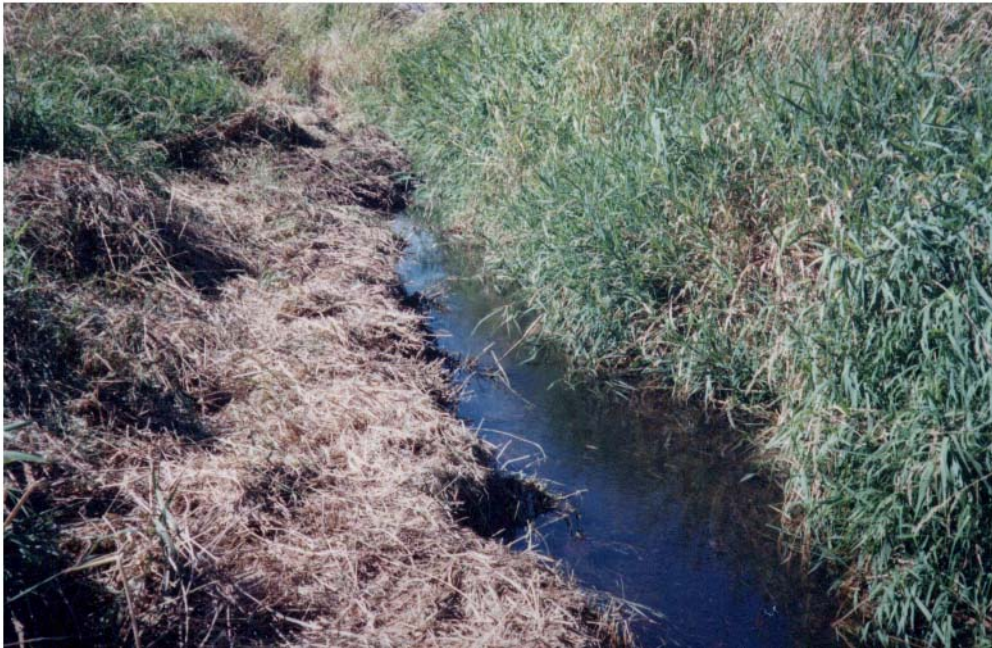
Photo 2: Reed Canary Grass was cut by hand with a scythe or gas powered brush cutters prior to excavation
