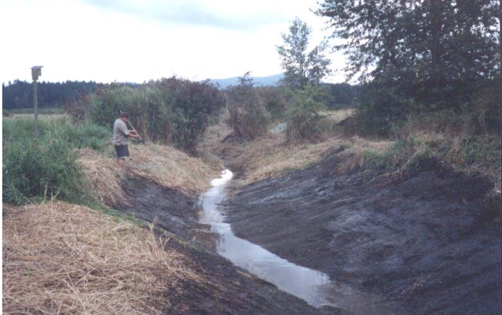
Photo 5: Following excavation, RCG cuttings were cast over the raw banks to retard its growth
